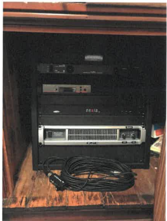
Existing sound system and amplifier controls.
