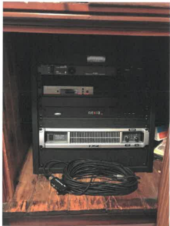
Existing sound system and amplifier controls.
