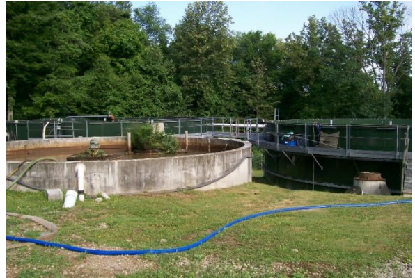
Penn E&R designed and installed an innovative water supply and treatment system for a resort in central Pennsylvania.
