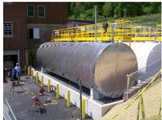
Penn E&R installed an AST after removing two leaking USTs from a health care facility.
