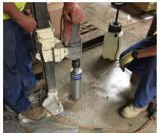
Penn E&R technicians drill through a concrete slab during a site investigation.
