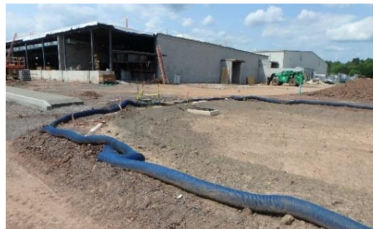
Filter socks are often used to trap sediment and control stormwater runoff at project sites.
