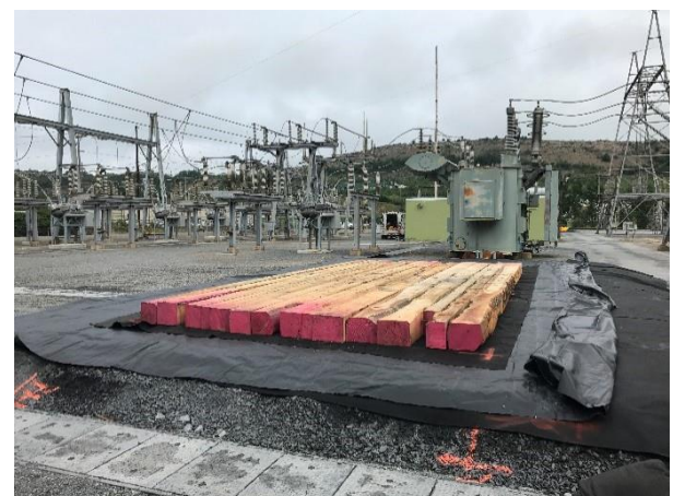
Penn E&R construction team installs temporary transformer storage containment pad for major utility client.
