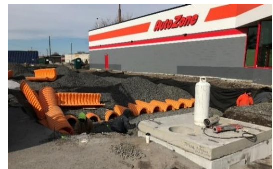
Stormwater management system installed below a retail store parking lot.
